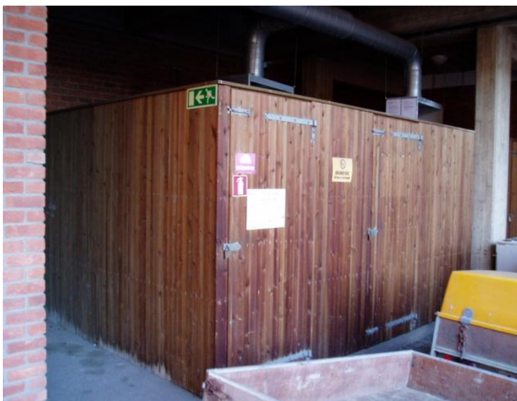
The shed with the waste tanks
