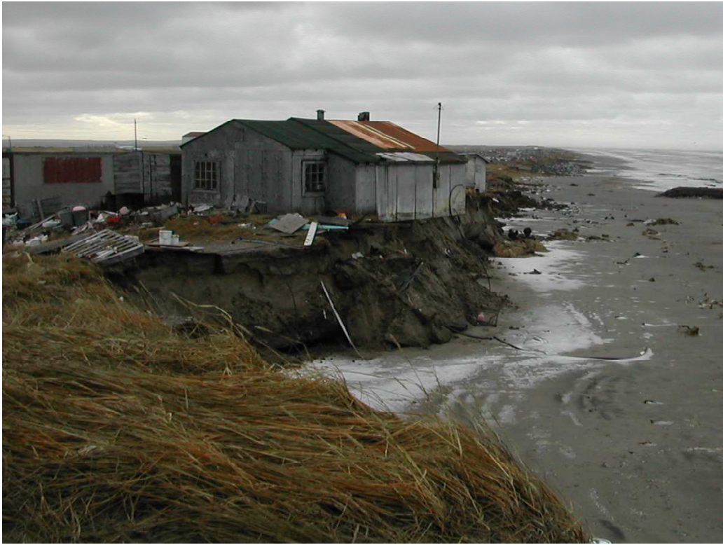
Figure 6: A residence in the native village of Shishmaref in Alaska showing the impact of wave action from the ET of Super Typhoon Tokage on a coast line that has lost permafrost. The buildings of the village have been relocated several times from such events. Courtesy of James Partain (NOAA Alaskan Region of the National Weather Service).
