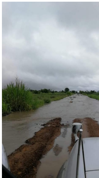
Figure 3.3: The road to Nwgelero Clinic after a heavy rainfall
