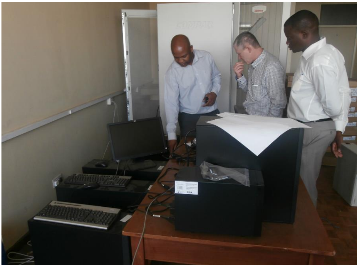
Figure 5 National server room hosting new DHIS 2 system on one of the machines
