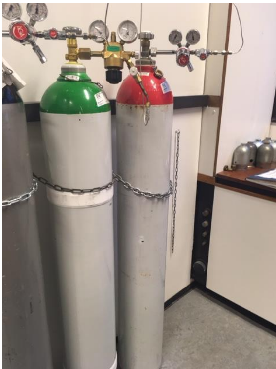
Bottles must be secured to the wall
